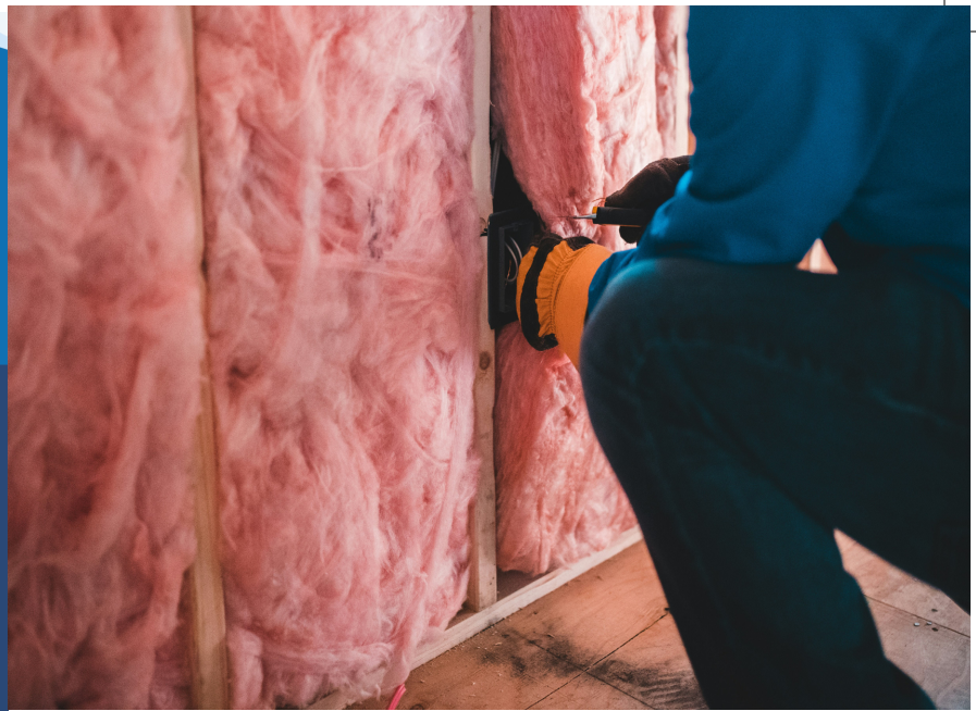
Without home insulation, even the best designed home will allow heat to transfer through walls, ceiling, and floors. Photo Source: Erik Mclean
